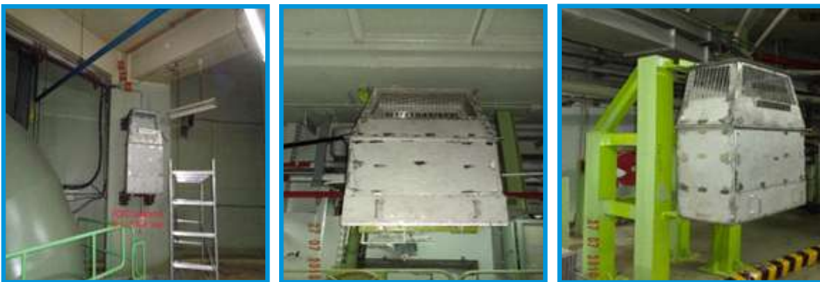
PCRDs installed at TAPS-3&4
