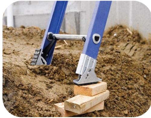
Improper placement of ladder on uneven surface
