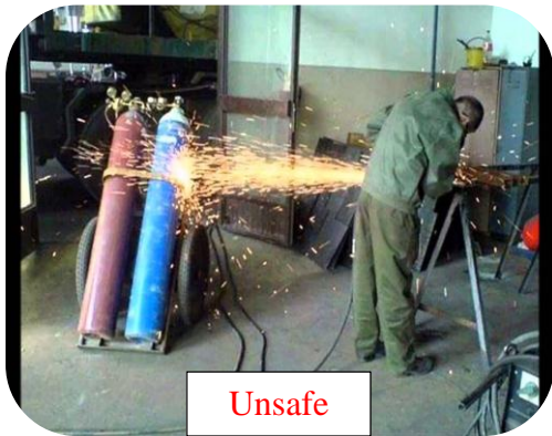
Gas Cylinders not properly placed & worker without proper PPE
