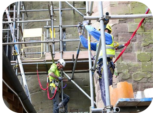
Wide and secured platform while working at height along with proper PPEs ensures safe working condition
