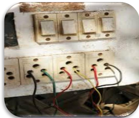
Unsafe Power Distribution Board
