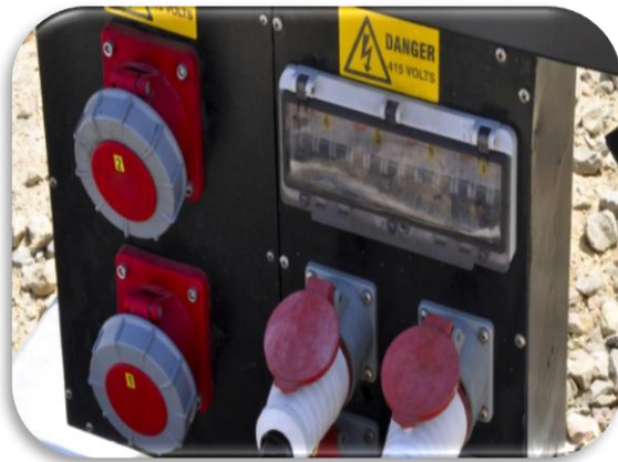
Safe Power Distribution Board
