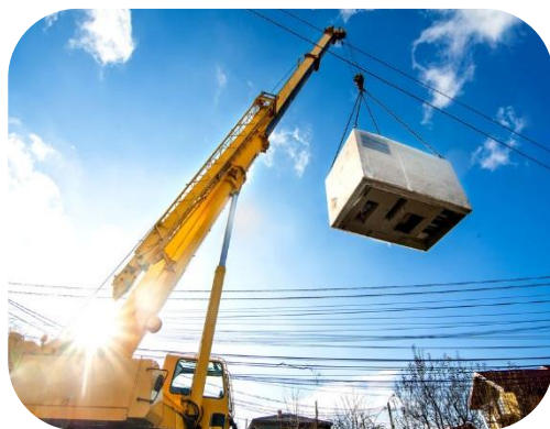
Insufficient clearance between crane boom and electric line
